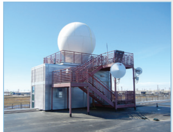
A newly installed X-SAPR operates from atop the Barrow Arctic Research Center in Alaska.
