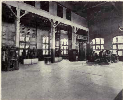
Interior Substation "B" Peoples Light Co. Davenport, Ia.
