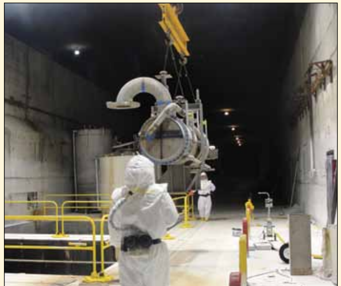
A heater is loaded into an open cell at U Canyon as work progresses to clear the deck of the facility.
