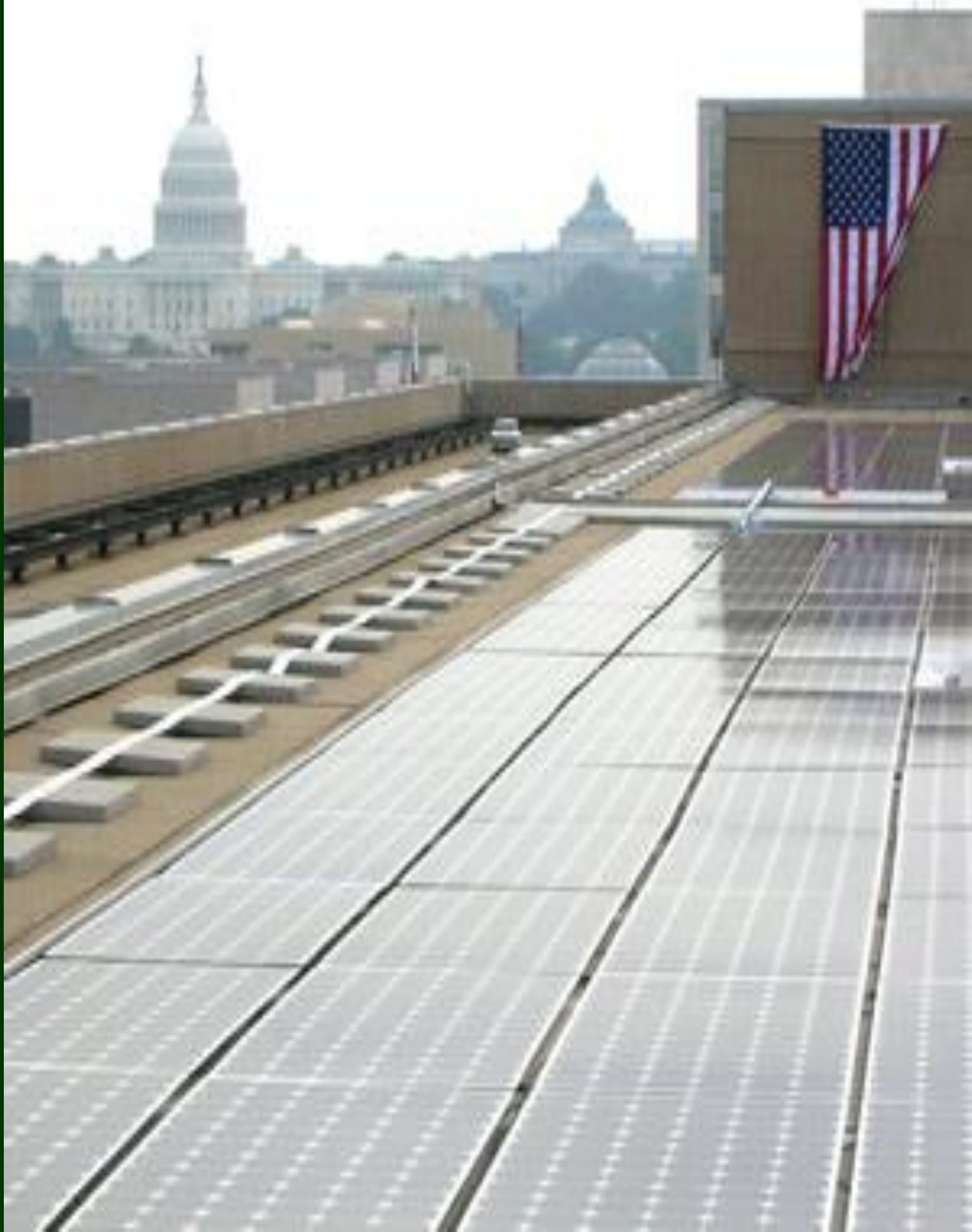
Solar panels on the roof of the Department of Energy's Forrestal Building in Washington, D.C.
