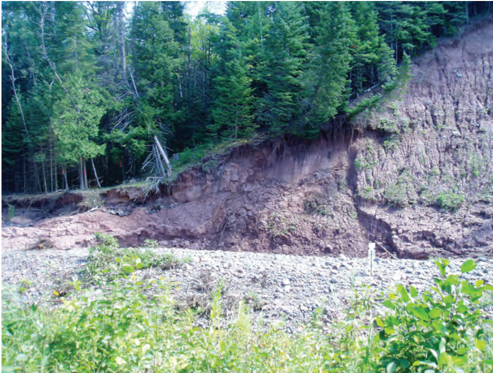
Figure 17. August 23, 2005 photo of failure at downstream end of bluff at site 14.4.
