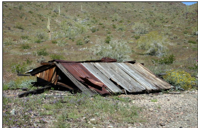
Figure 3-10. Collapsed Miner's Shack located in the Northern Cibola Region
