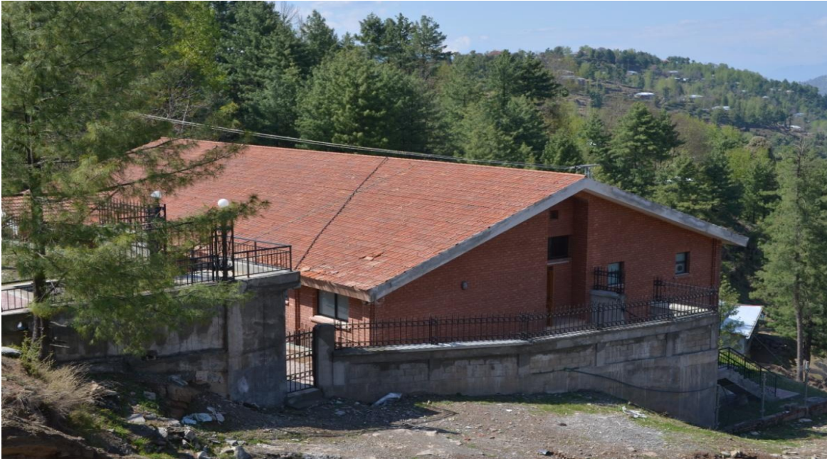
This health-care facility in Neela But, Bagh, is not in use and has deteriorated since it was turned over to the Government of Pakistan. As shown above, roof tiles are damaged. (Photo by OIG, April 16, 2012)
