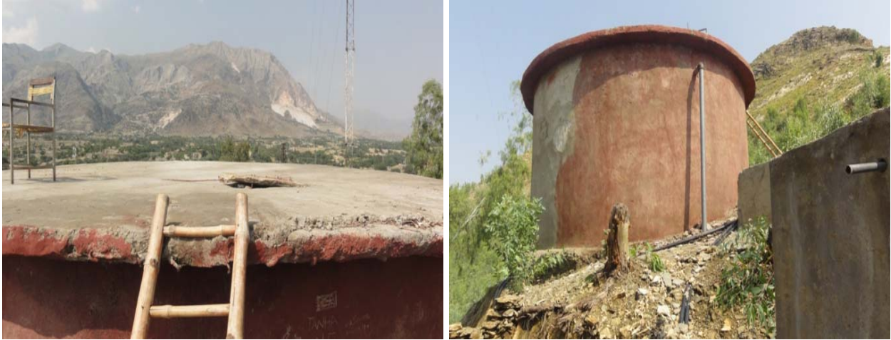
This program-funded tank, shown from two angles, delivers water to a village. (Photos by OIG, October 2011)
