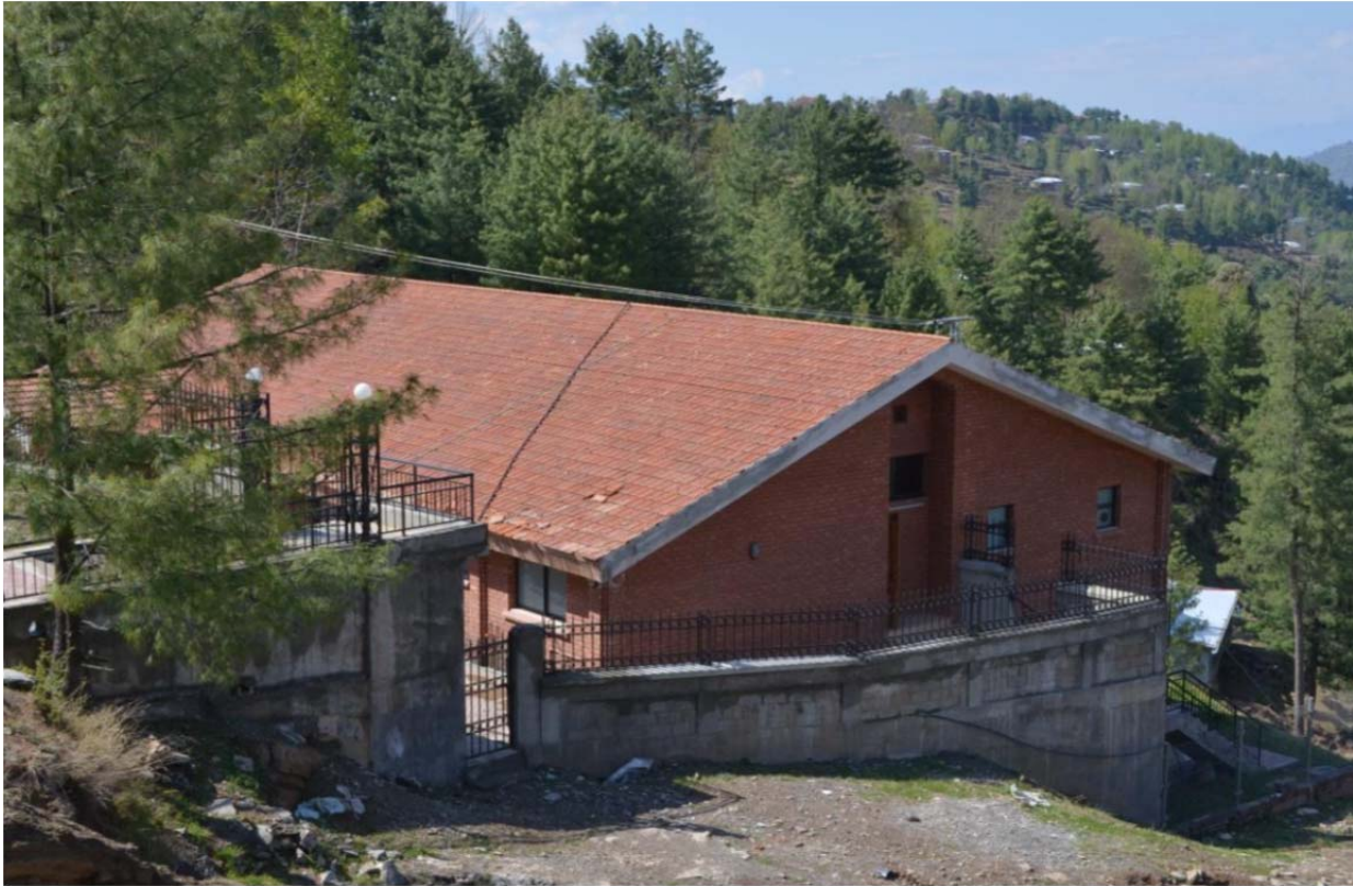
This health-care facility in Bagh is not in use and has deteriorated since it was turned over to the Government of Pakistan. As shown above, roof tiles are damaged. (Photo by OIG, April 16, 2012)
