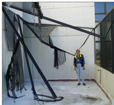
AOML Deputy Director Judy Gray inspects damage to a screened patio area at AOML after Hurricane Wilma's passage on October 24th.
