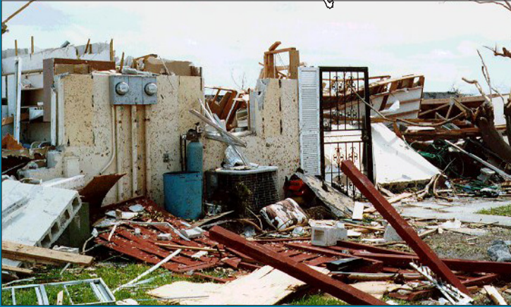
Front view of the Naranja Lakes townhome where AOML electronics technician Michael Shoemaker spent the early morning hours of August 24, 1992 with his mother. The two survived by climbing out of the rubble and finding shelter at a neighbor's house as Andrew's eyewall passed overhead.
