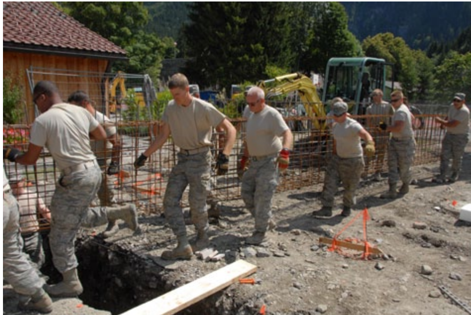
Airmen of the 184th Civil Engineer Squadron put rebar in place for the footings that will hold a new pavilion during a mission in Oberammergau, Germany. Photo by Tech. Sgt. Justin Jacobs, 184th Public Affairs
