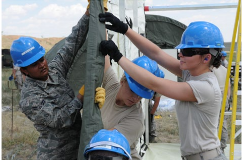
Airman 1st Class Binny Muncrief, Airman 1st Class Chelsey Thompson and Airman 1st Class Tiffany Golden assemble a deployable structure as the 134th Air Control Squadron constructs an operational tent city at Fort Carson, Colo., during a field training mission.
