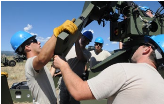
Senior Airman Tim Mercer, Staff Sgt. Matt Gefaller, Staff Sgt. Everardo Lopez and Staff Sgt. Nathan Morgan, RF Transmission Shop, assemble the Quad-Band Large Aperture Antenna Dish on an AN/TSC-179 Ground Multiband Terminal, which provides all the long haul (satellite) communications.
