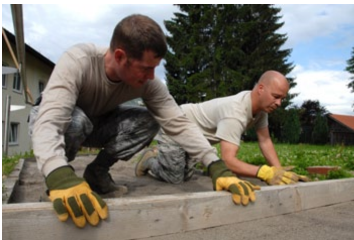
Staff Sgt. Zach Whitener, 184th Communications Flight, and Tech. Sgt. Karey Haukom, 184th Civil Engineer Squadron, resurface a walkway at the NATO school on base. Photo by Tech. Sgt. Justin Jacobs
