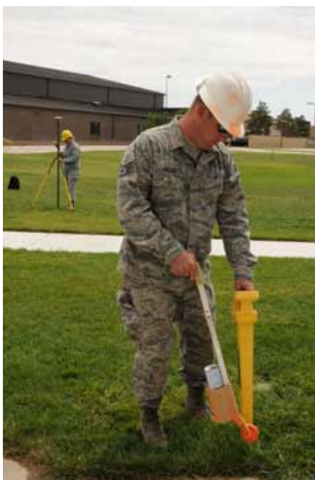
Left: Staff Sgt. John Pollard tracks and marks cable locations with orange spray paint, indicating where communications lines are buried.
