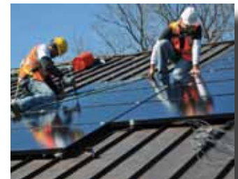
DoD is using Recovery Act-funds for this solar panel efficiency project.
