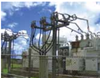
DoD IG inspected Guam's Harmon Substation, 115 KV Transformer Bank.
