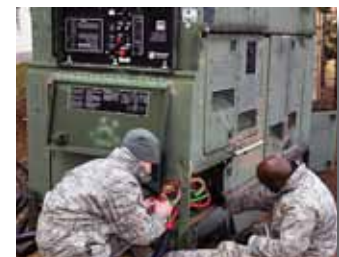
AFAA evaluated Air Force emergency and standby generators.
