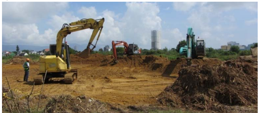
Clearing and grading the thermal desorption treatment pile area (Photo: CDM Smith)
