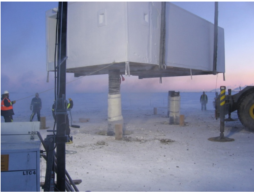
Fig. 8—Installation of the observatory building on top of pilings used to support the structure in permafrost.
