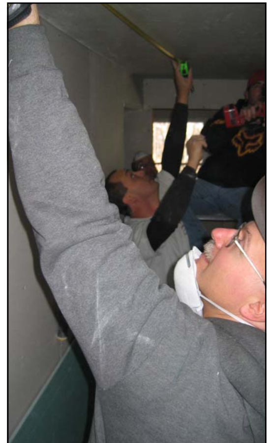
Master Sgts. George Blackwell and Mike Murphy measure a ceiling where drywall was installed.
