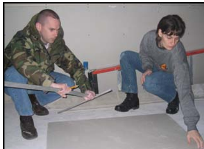
Tech. Sgt. Joe Jones and 1st Lt. Teri Hunter measure drywall that was installed in a master bedroom.
