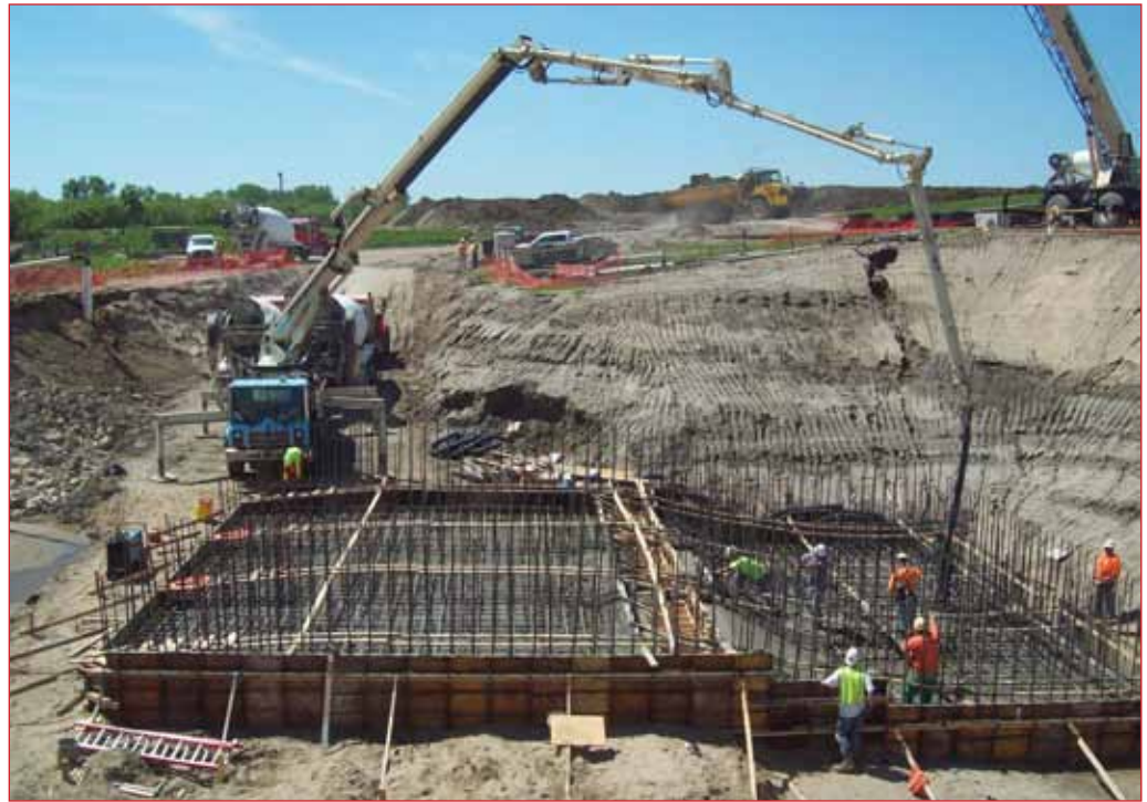
The foundation is poured for a pump station on the Chain of Rocks levee April 18. The pump station is part of the federal project to restore the Metro East levees to their original authorized level of protection.
