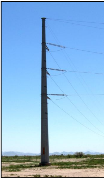
Photograph 2-2 Example of a Metal Monopole
