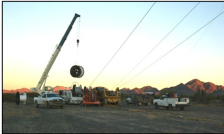
Photograph 2-5 Example of Tensioning Equipment
