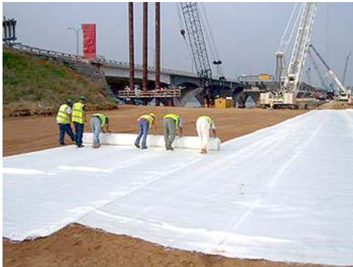
Crews are installing geotextiles at the Woodrow Wilson Bridge site in Washington, D.C. The process looks a little like laying wall-to-wall carpet.
