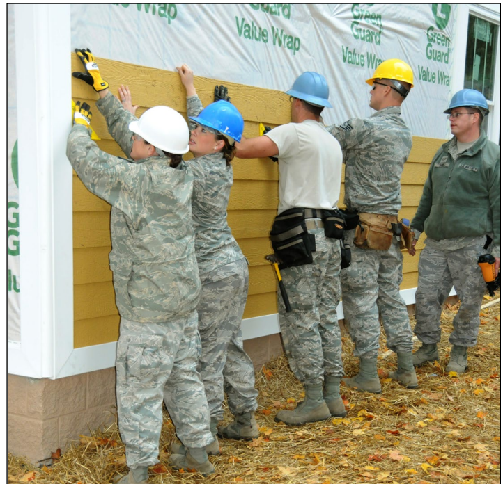
Airmen with the 183rd Civil Engineering Squadron, 183rd Fighter Wing help construct a home with Habitat for Humanity through an Innovative Readiness Training project in Springfield, Oct. 13. The project is scheduled for three years and the 183rd CES will help build numerous homes in Sangamon County during that time. (Air National Guard photo by Tech. Sgt. Andria Sapp/Released)
