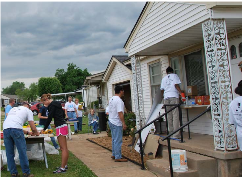
Unit members work on making repairs for Mrs Howard's home during the May UTA weekend.
