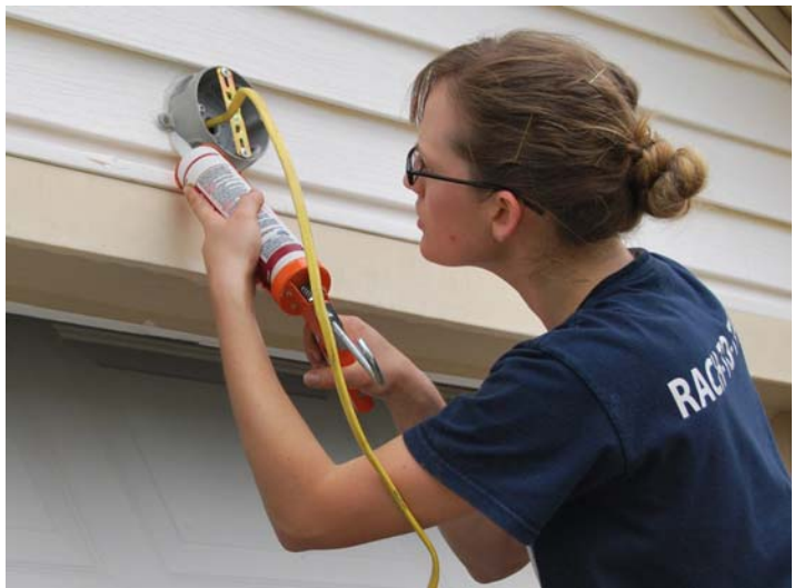
A new security light above the garage gives Mrs. Howard peace of mind.
