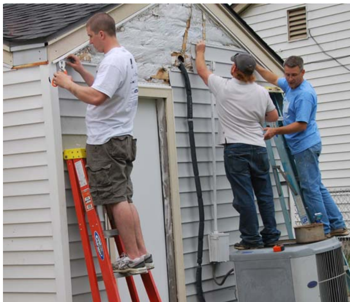
Hail-damaged siding had to be removed and replaced.
