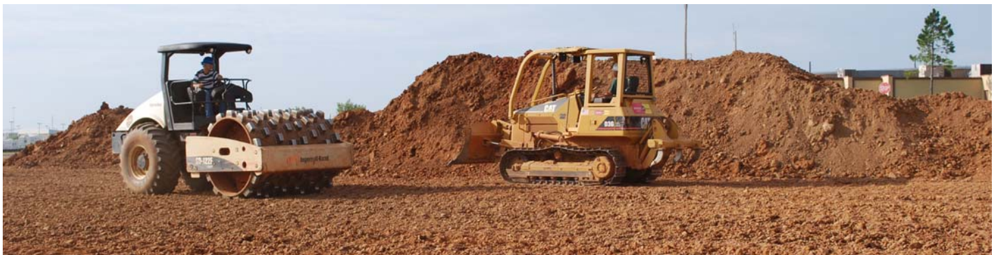
The crews were back at work on the site after the groundbreaking ceremony.
