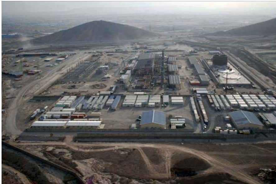
A 105-megawatt power plant and supporting structures under construction in Kabul. (Photograph by implementing partner.)
