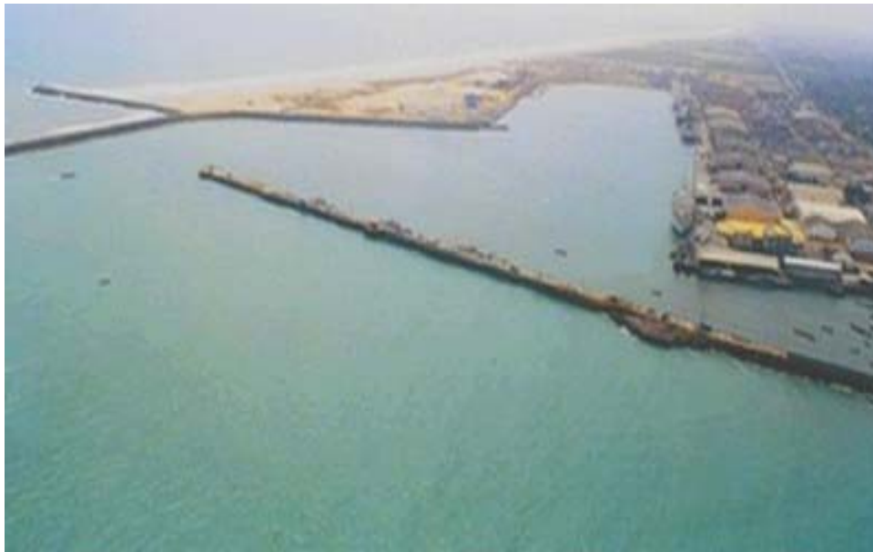
MCC activities at the Port of Cotonou in Benin include extending the jetty (top left) and constructing of a new wharf to accommodate additional containerized merchant marine vessels. The left side of the U-shaped harbor will become the new South wharf. (Photograph courtesy of Port of Cotonou Web site.)
