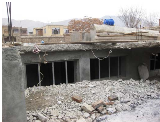
The program purchased materials to rebuild a home for 19 family members in Kabul after an aerial bombing destroyed the building during a military operation. (Photograph by OIG.)
