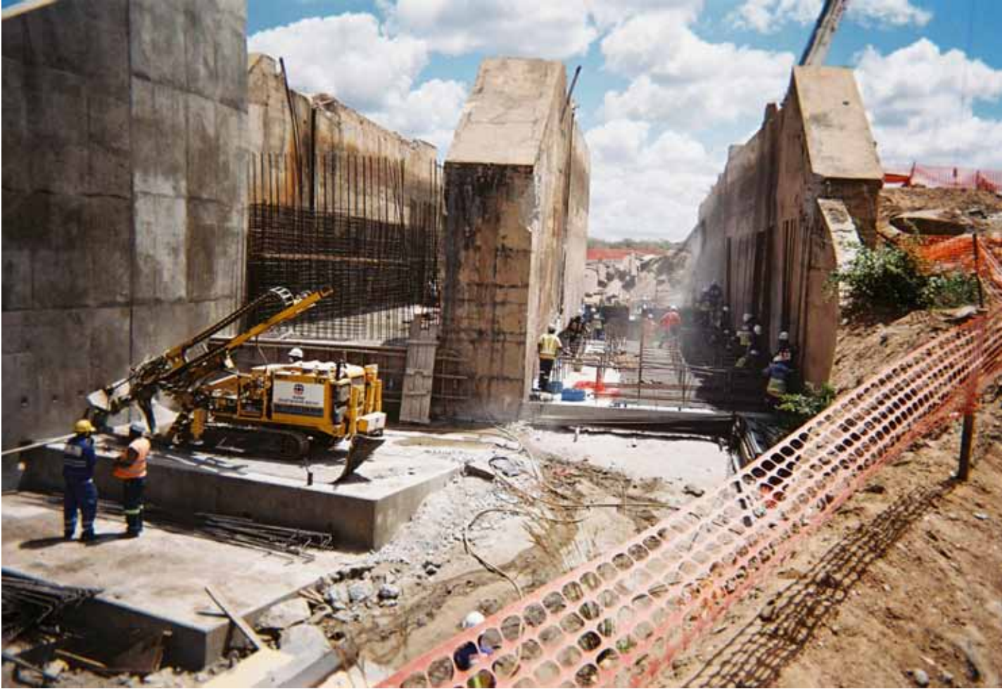
Construction on the Nacala Dam Rehabilitation project in Mozambique is currently underway.
