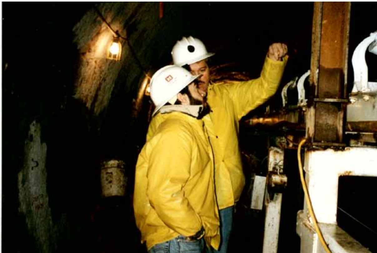
Sean Dolan (left) and Frank Fedele discuss a piece of machinery in the tunnel being constructed as part of the Town Brook Local Protection Project in Quincy, Mass., in this photo taken in the 1990's.
