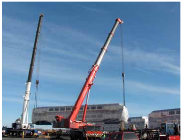
New MBTA double-decker railcar is lifted off barge at the New Bedford Superfund Treatment Plant.
