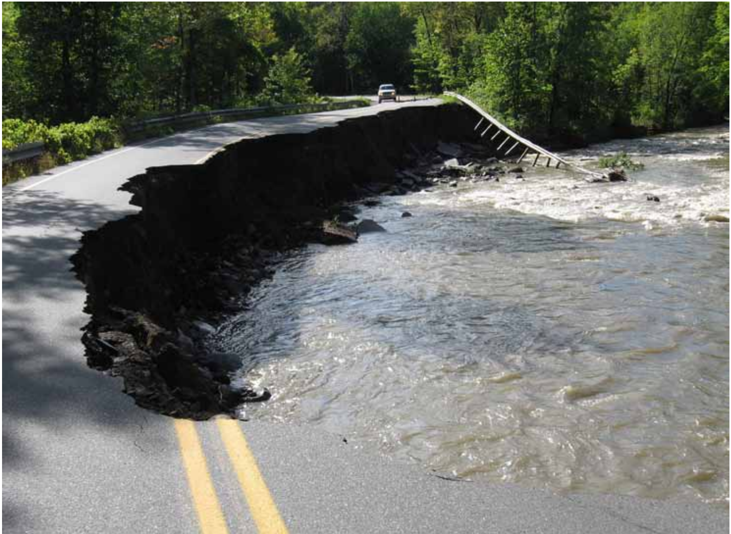
Hurricane Irene washed out many roads like the one above, causing delays hauling out material from Union Village Dam. Despite the challenges brought on by the storm, the District was able to complete the project on time. File photo
