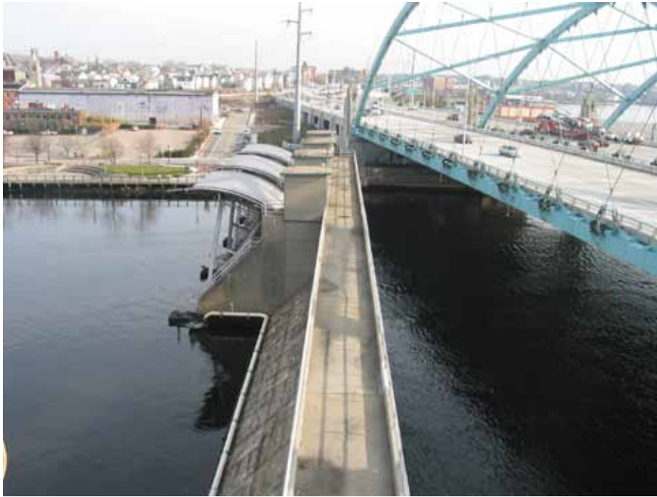
The Fox Point Hurricane Barrier in Providence, R.I. operates during the storm event.
