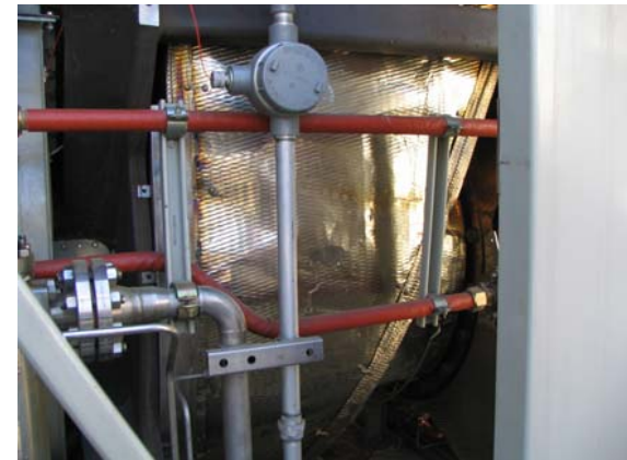
Mercury 50 Turbine Section
