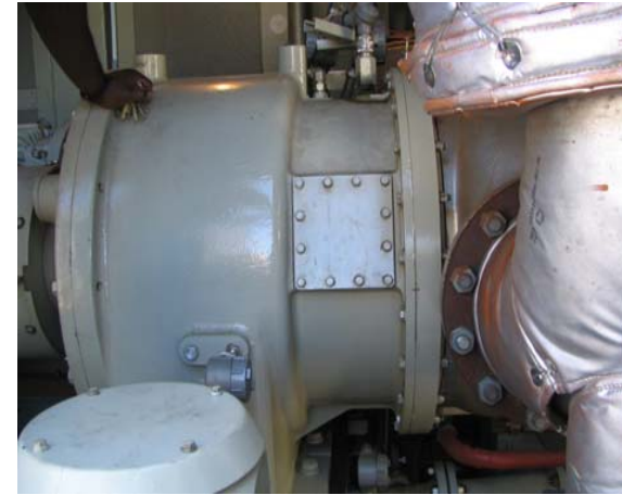
Mercury 50 Compressor Section
