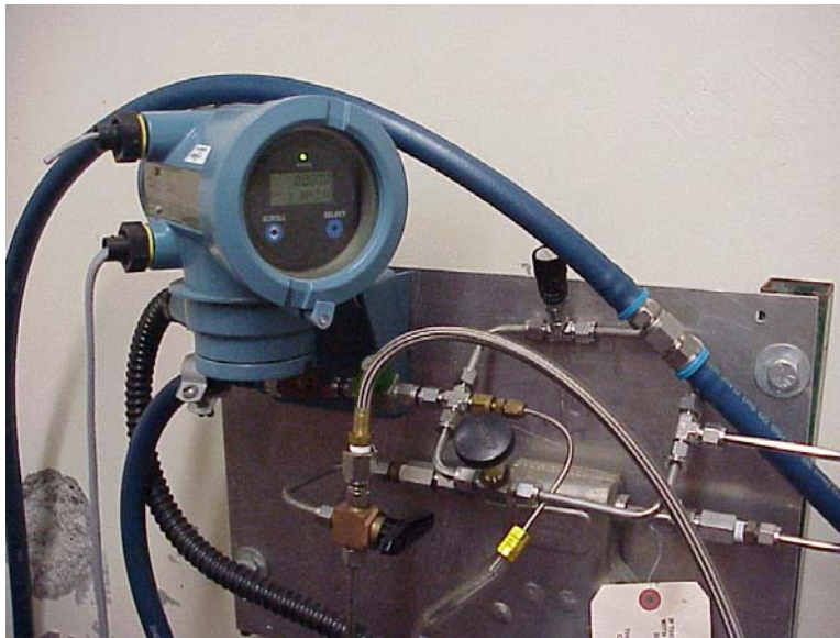
Figure 10. Fuel Flow Control and Metering.
