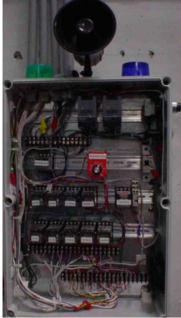
Figure 12: Main Box for Relays/Controls for Safety System
