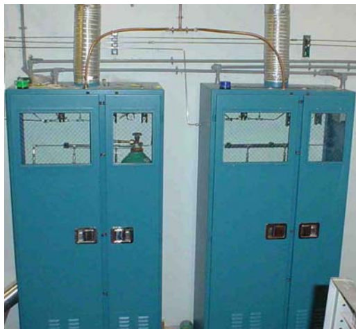
Figure 5: Gas Storage Cabinets for Hydrogen and Carbon Monoxide Gas
