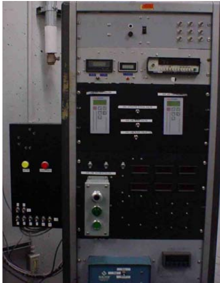
Figure 13: Main Control Panel in Control Room
