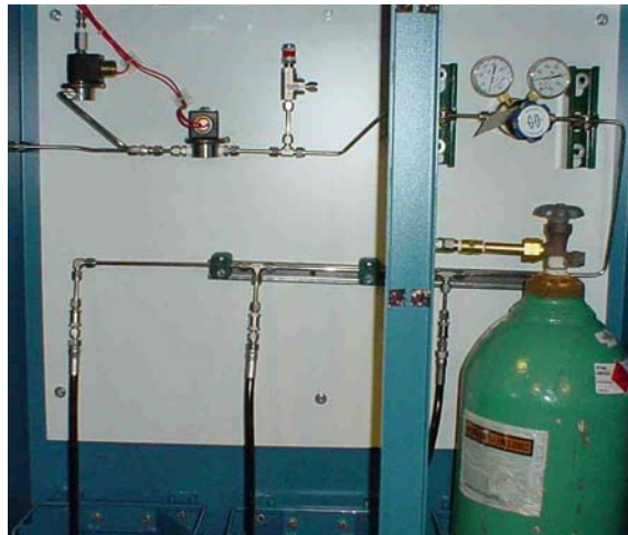
Figure 7: Bottle Valving and Controls for Hydrogen and Carbon Monoxide
