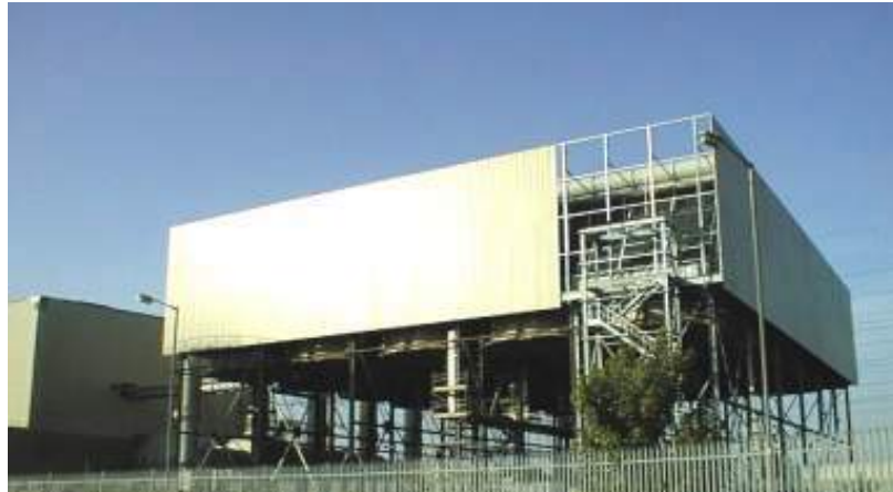
Air Cooled Condenser
