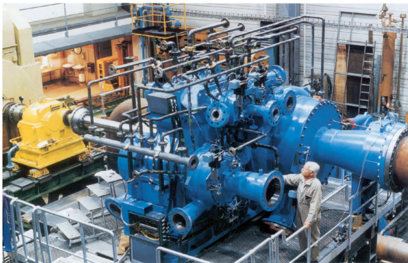
Compressor Unit during test run in MAN GHH BORSIG test bed
