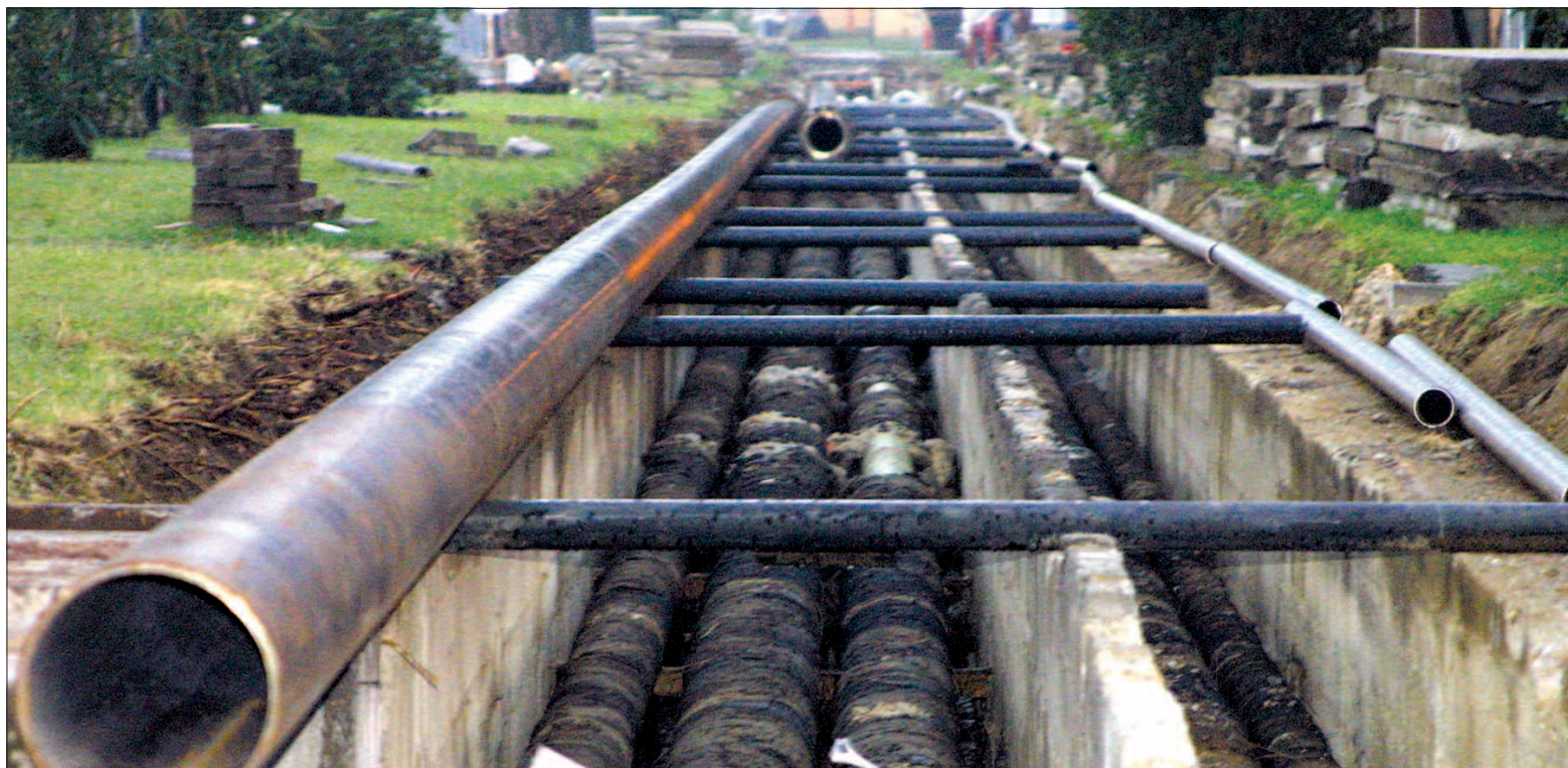
Trenches filled with pipes have dominated the Caserma Ederle landscape for months. Construction projects will continue on the post, in Villaggio and at Longare for many years to come. However, the new facilities will provide better living conditions throughout the community.
