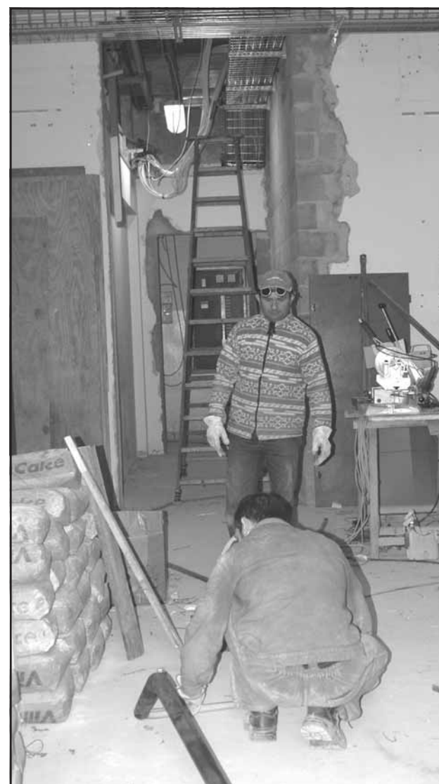
Contractors work on renovations to AFN South facilities. With a cost of $1.65 million, the work brings the facility into compliance with Italian building codes, which are enforced at the national and local levels, according to Lt. Col. Donald Ross, AFNS commander.
