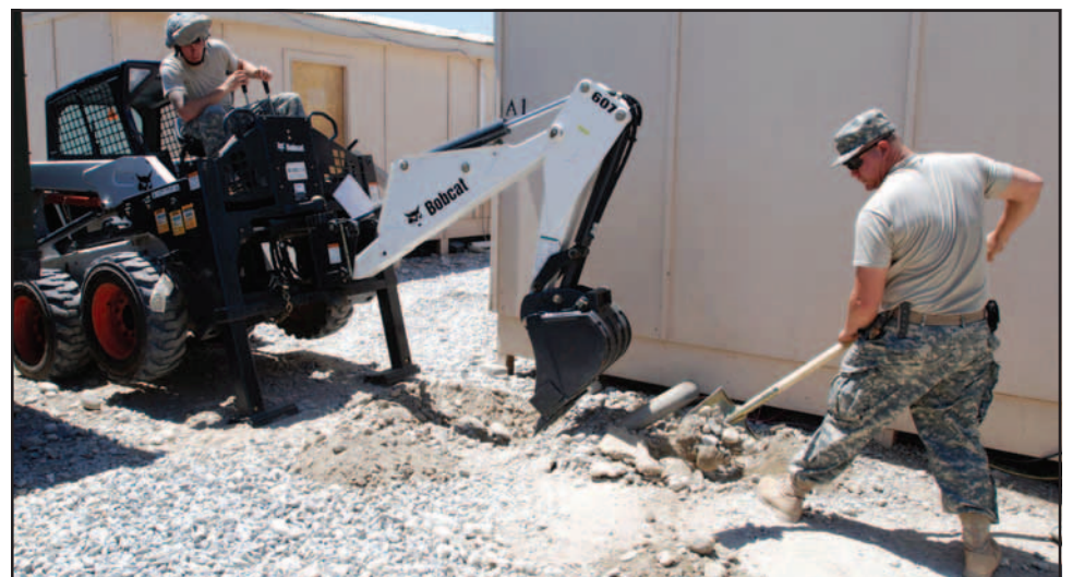
Pvt. Ben Williams (left), 76th Engineer Company and Sgt. Christopher Masterson (right); Charlie Company, 173d Special Troops Battalion, dig a trench to bury Internet lines in the combat teams tactical operations center June 4 at Jalalabad Airfield.
