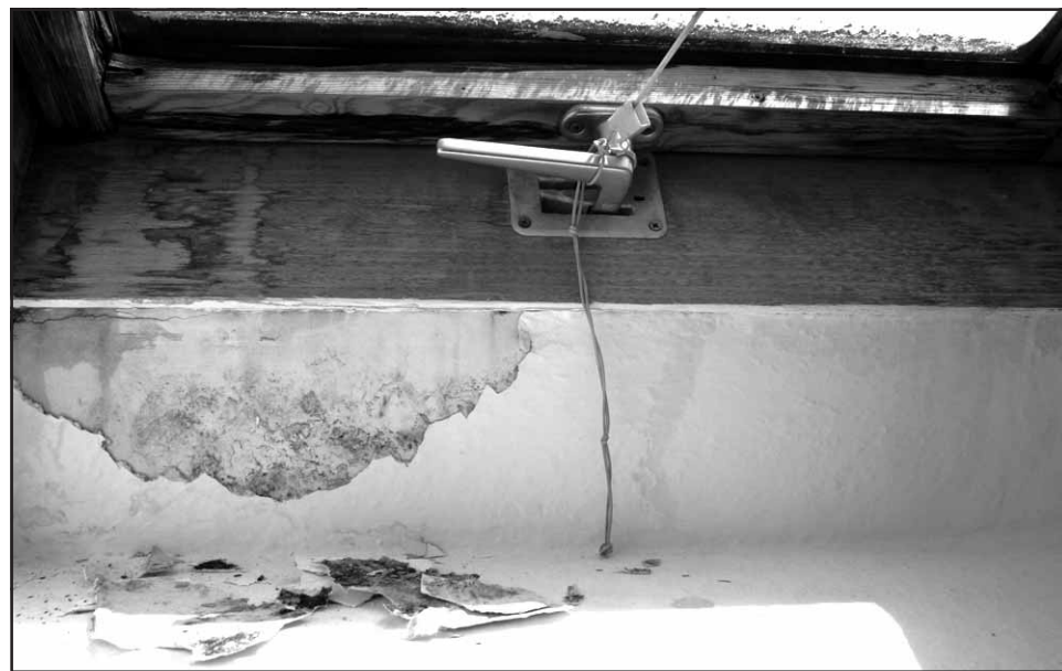
Moisture let in by leaky windows is a leading cause of mold.
