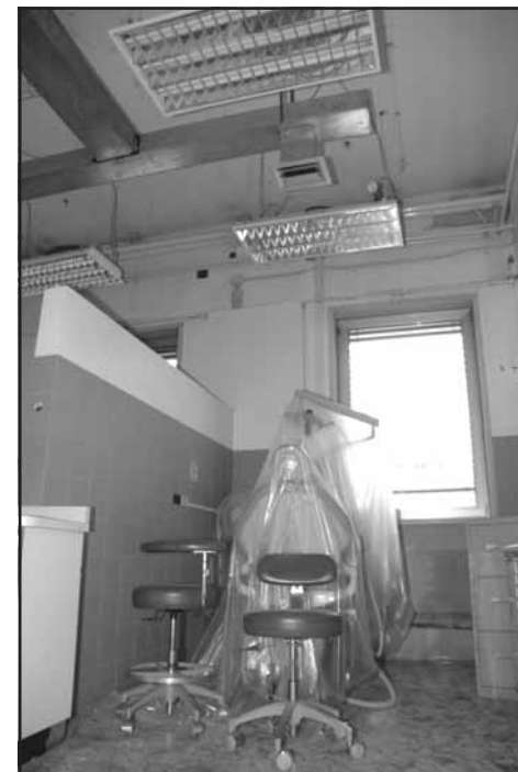
Dental chairs are covered with plastic and the ceiling is removed, exposing wires and ducts. The heating and cooling system and electric in the clinic are being updated over the next few months to provide a lighter clinic and better climate control.
