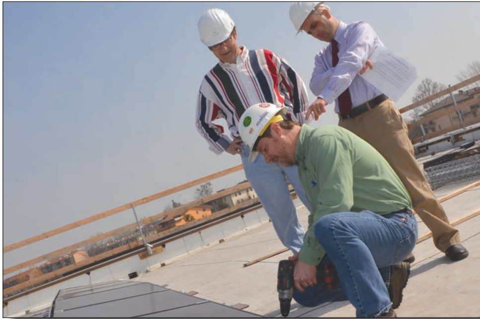
Ron Pinkoski, Directorate of Public Works Environmental Protection specialist, checks the installation of a fastener on a solar panel on the top of the commissary, while Greg Vallery, left, and Mark McWilliams look on. The panels placed on top of post buildings will help save around $1.1 million per year.
