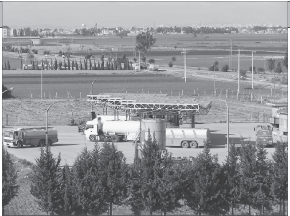
Trucks pull in to the JP8 truck-loading facility in Adana, Turkey.
