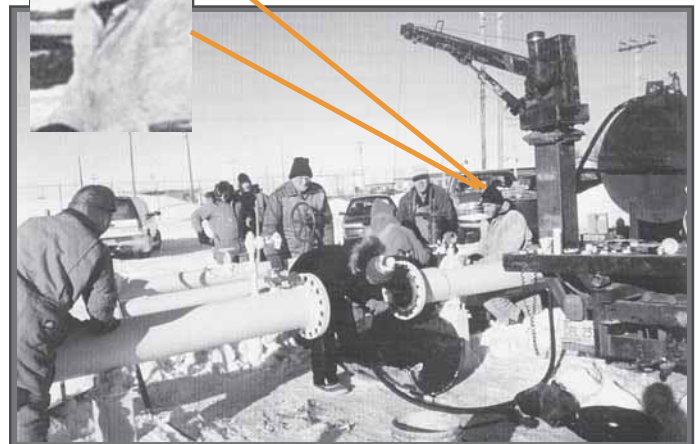
Crews work in sub-zero temperatures to free a stuck 'pig' from the pipeline at DFSP Grand Forks in 1996. Mac McIntosh is standing center; Dave Kovar is out of view. (Photo by Bill Pulley)
