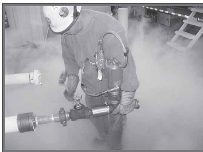
An employee checks the safety valves on the nitrogen hookups used to propel the “pig” and “pickle” the pipeline Oct. 3.
