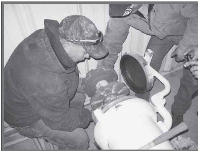
The pipeline inspection gauge is loaded at Defense Fuel Support Point Grand Forks in preparation for the last pipeline delivery to Grand Forks Air Force Base Oct. 3.
