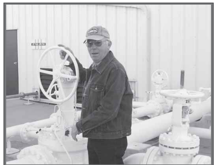
He’s got it coming and going Bill Pulley, a former employee at the DFSP, opens a valve at the DFSP to start the final delivery of fuel to the air base Oct.3. As a young airman at Grand Forks AFB in 1959, Pulley received the first pipeline delivery from DFSP Grand Forks.
