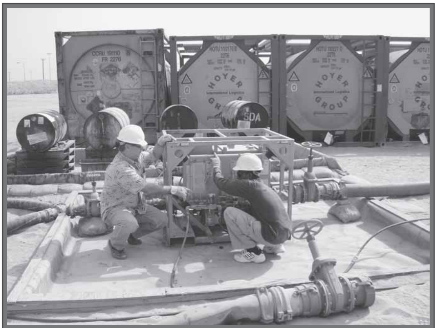
Quality Assurance Representative KO. Williamson inspects a Hammond Injector at a truck fill stand in Kuwait. Behind him are the bulk Fuel System Icing Inhibitor storage containers.
