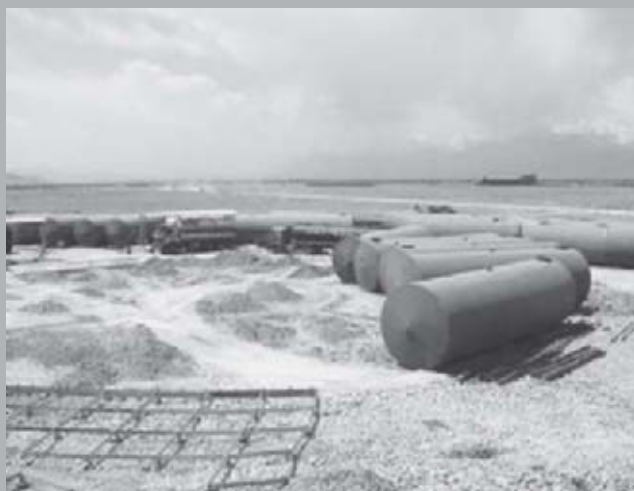
Down-loading and up-loading points at the fuel facility under construction in Afghanistan.
