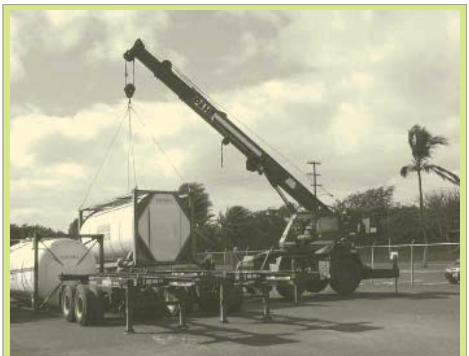
A crane loads the empty Iso-containers onto a chassis at Hickam Air Force Base, Hawaii, for movement to Pearl Harbor where they will be filled.
