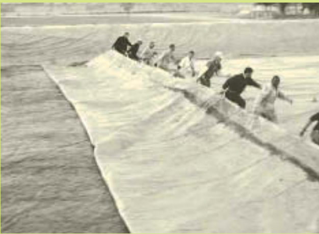
As the last major step for shutting down fuel operations at 'K2', workers folded the multi-thousand-pound fuel bladder back and forth to recover the unattainable fuel from the 120,000 gallon fuel bladder.
