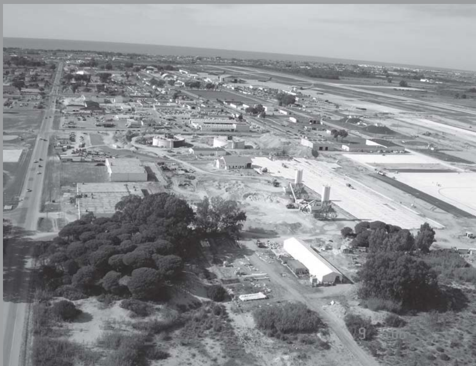
In this aerial view of U.S. Naval Station Rota, construction for the Strategic Airlift Enroute System is underway. The Enroute system will help the U.S. Air Force meet one of its core competencies, Rapid Global Mobility. The construction project will add seven miles of pipeline, triple the hydrant tank capacity, and increase the number of fuel hydrant spots for aircraft refueling. The project will also help support the expanding missions of American and NATO forces.
