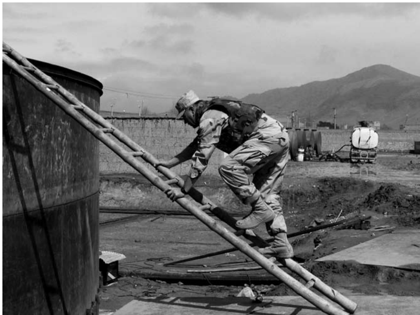
Col. Michael Giroux, director of DESC's Facilities and Distribution Management commodity business unit, scales a bamboo ladder to inspect progress on a fuel storage tank being manually constructed in Kabul, Afghanistan. (Photo by Col. Dave Rohrer.)
