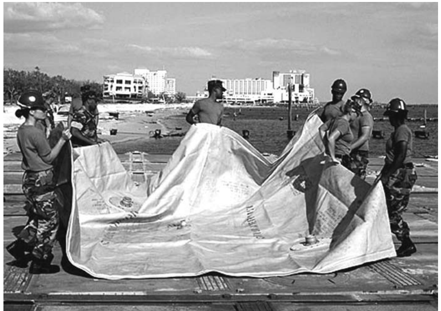
U.S. Navy Seabees from Amphibious Construction Battalion 2 conduct relief operations as they lay out the fuel bladder on the beach of Biloxi, Miss., in support of Hurricane Katrina Relief efforts on Sept. 6, 2005. U.S. Navy photo by Petty Officer 2nd Class Michael Sandberg
