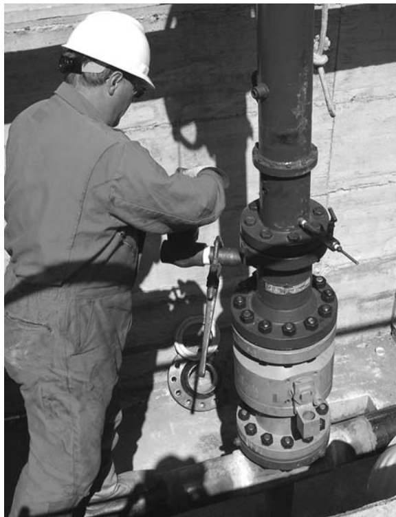
As part of the hot tap procedure, the pipeline cutting assembly is being assembled.
