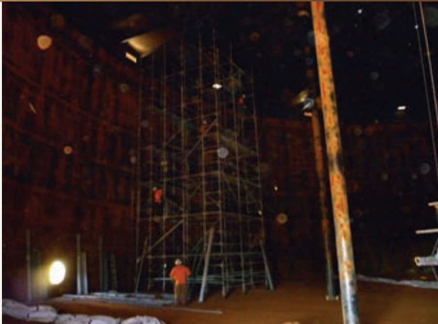
Repairs underway inside a fuel storage tank were funded through Defense Logistics Agency Energy's Sustainment, Restoration and Modernization funding process. Photo courtesy of DLA Energy Americas.
