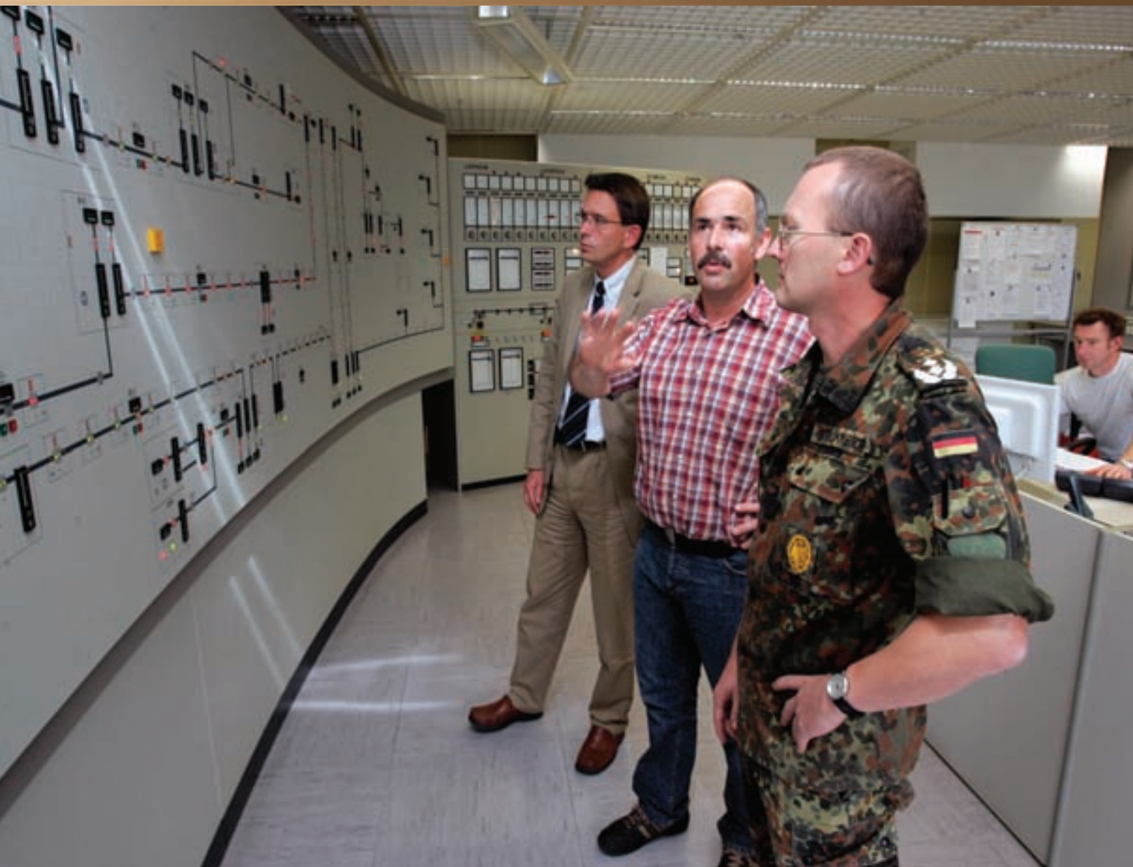
Central European Pipeline System Dispatcher Harald Schoefer, center, explains an automated board used to track pipeline operations to Joachim Elfner, head of the Southern German CEPS, left, and a German soldier. Photo courtesy of NATO.
