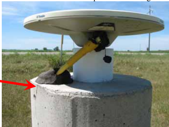
Figure 5 – view of pillar monument (note the crack that has developed near conduit location)
