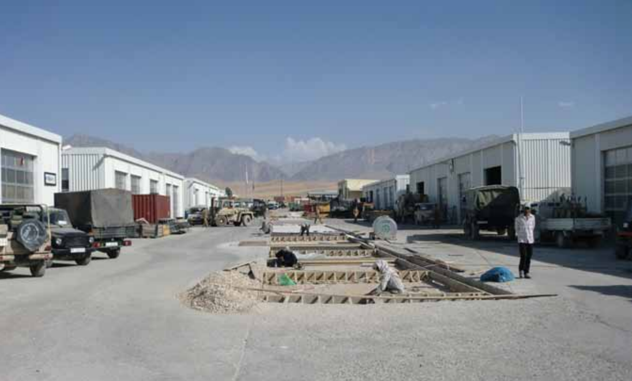
Construction work is conducted as part of the ongoing upgrade of this main vehicle maintenance facility, which houses work pits and vehicle shelters at an operating base in Afghanistan.
