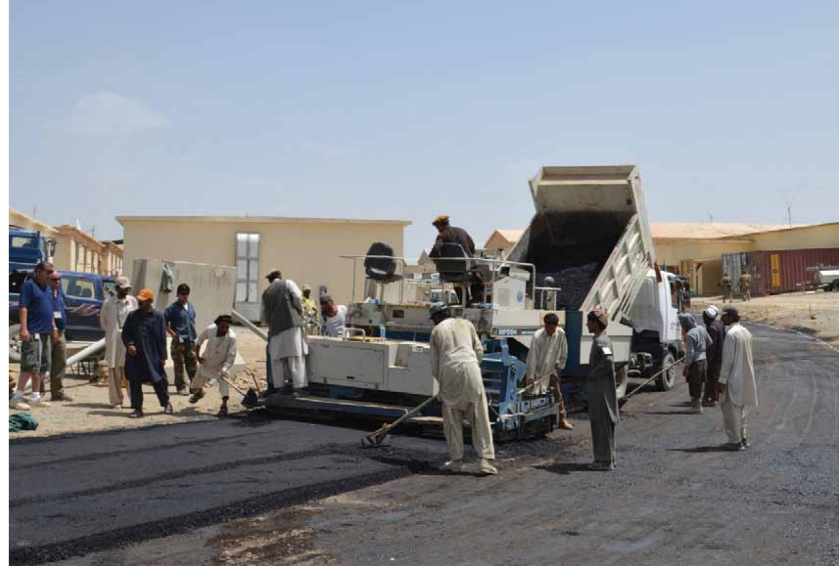
Afghan workers spread asphalt across a new road at Forward Operating Base Sharana. To help stimulate the economy and grow a skilled workforce in Afghanistan, the 243d Construction Management Team, Task Force Sword, follows the Afghan First policy when selecting contractors for jobs. (Photo by SPC David Huddleston)
