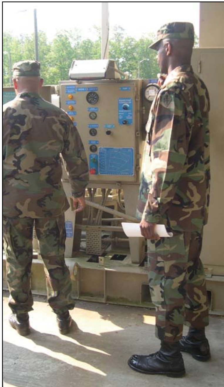
At an Inland Petroleum Distribution System site, Soldiers inventory components of an 800-gallon-per-minute mainline pump.
