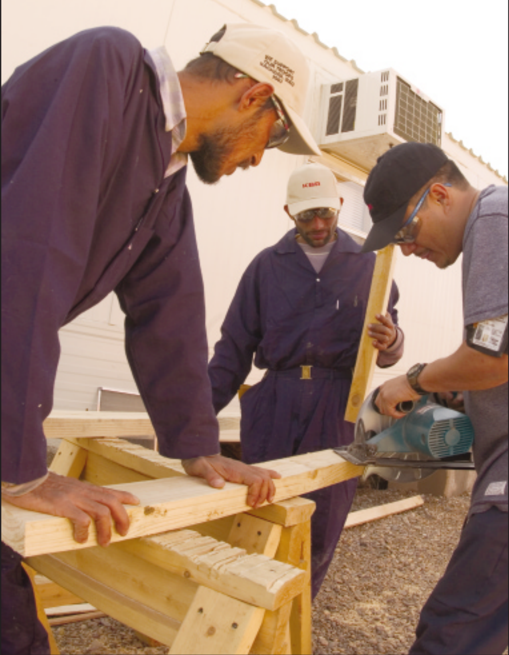
A KBR employee demonstrates proper sawing techniques to two Iraqi laborers as they construct a new military camp near Baghdad.
